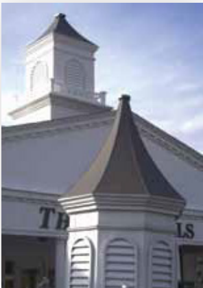
Old cupola in lower corner and new RF Friendly cupola in place on roof
